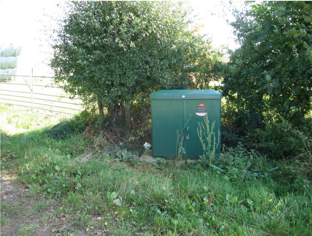
Photograph 3.2: An Existing CP Transformer Rectifier Cabinet
